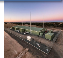
BESS 1) with grid-forming function
